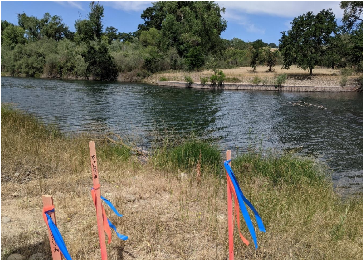
Figure 9. Photopoint 5a. PPT 5 faces northwest and is located on the left bank at the old bridge abutment. Photo shows the bridge abutment and portion of river where submerged I-beams are located.
